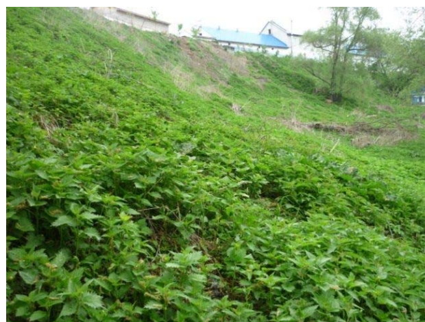
Fig.2 The landslide shape of a slope.
